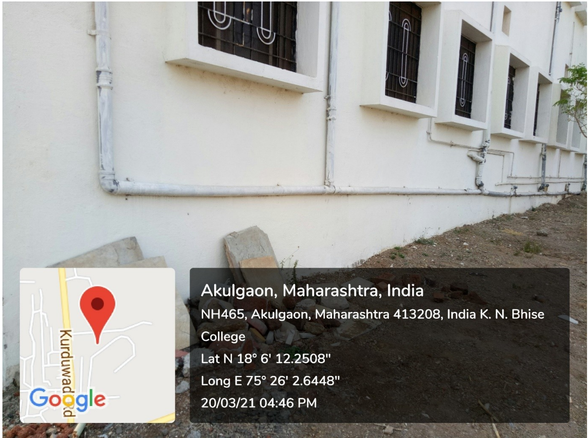
Hazardous Chemical Wastage Pipeline
