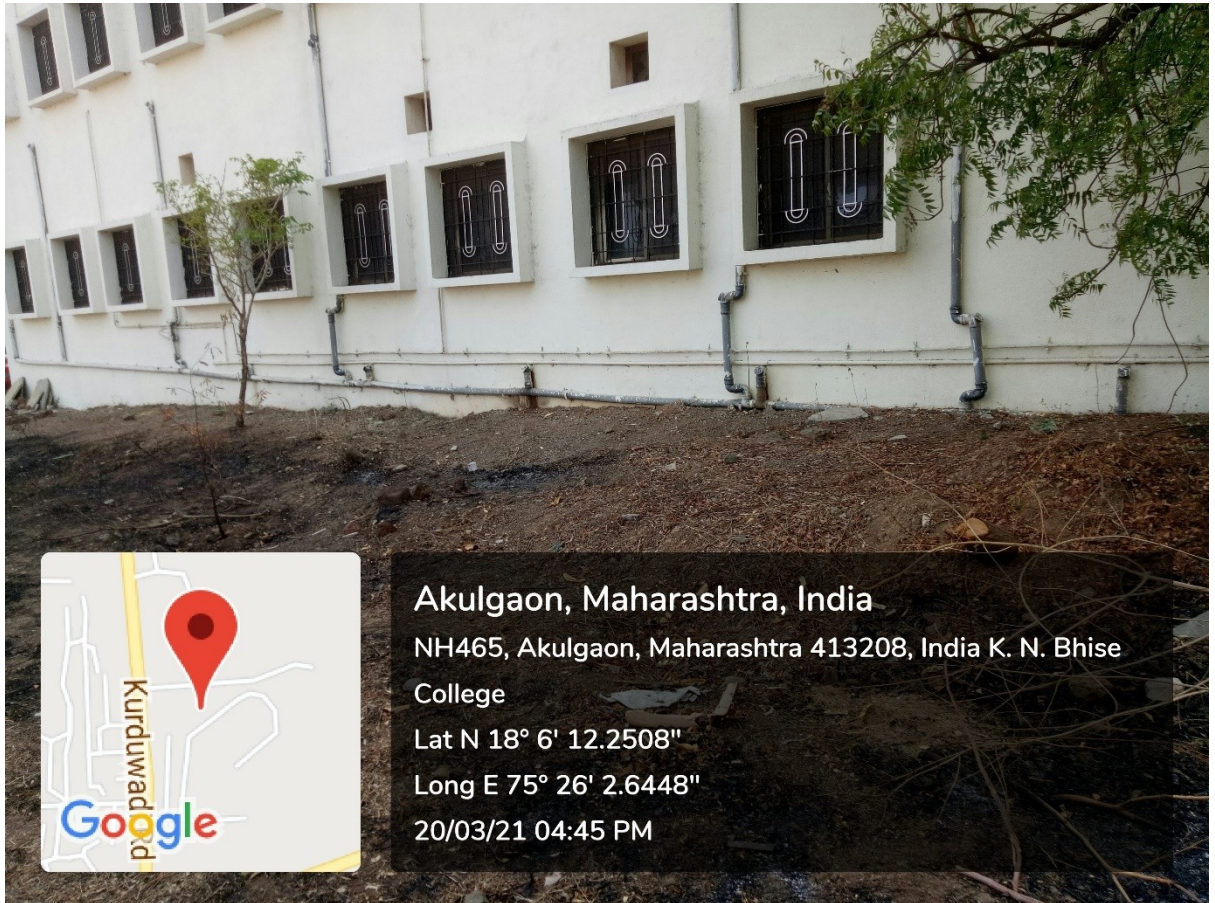
Hazardous Chemical Wastage Pipeline
