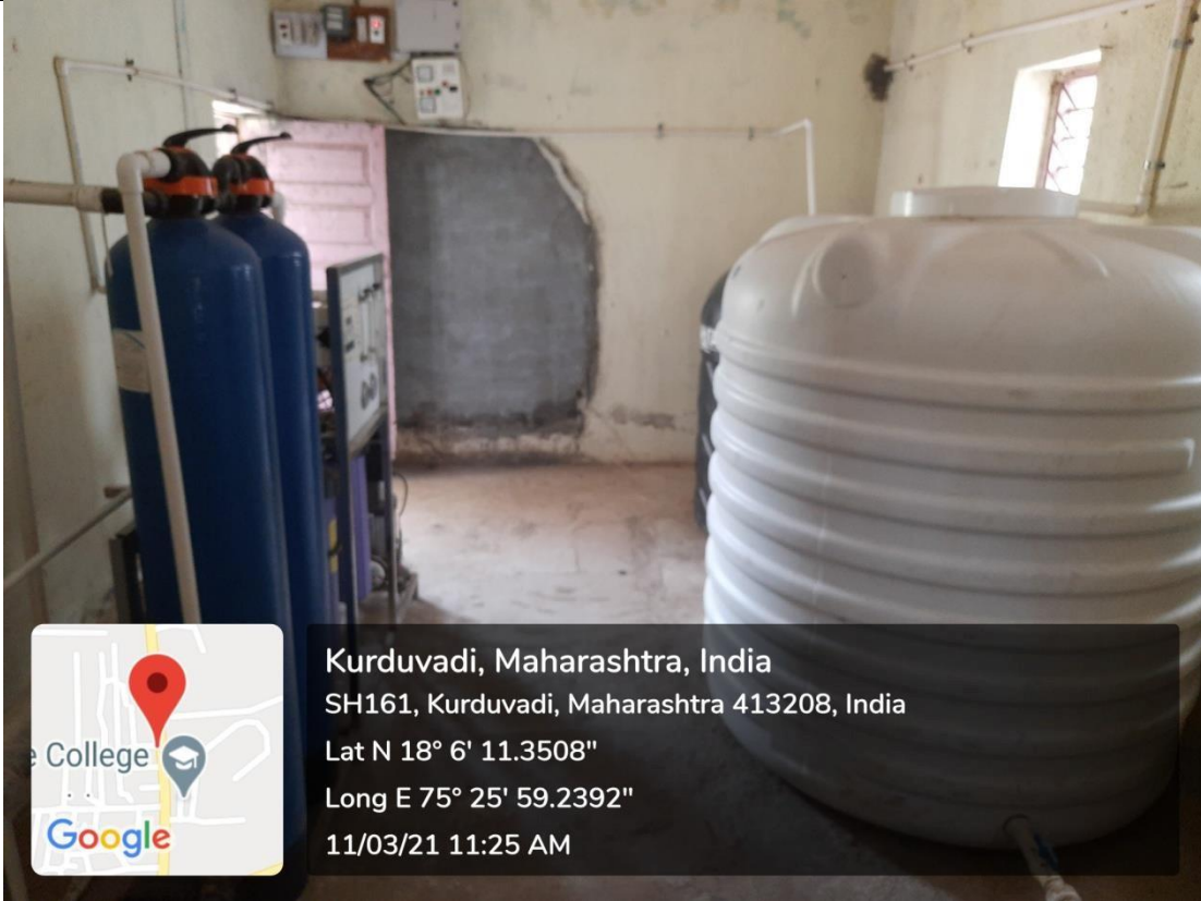
R.O. Water Plant
